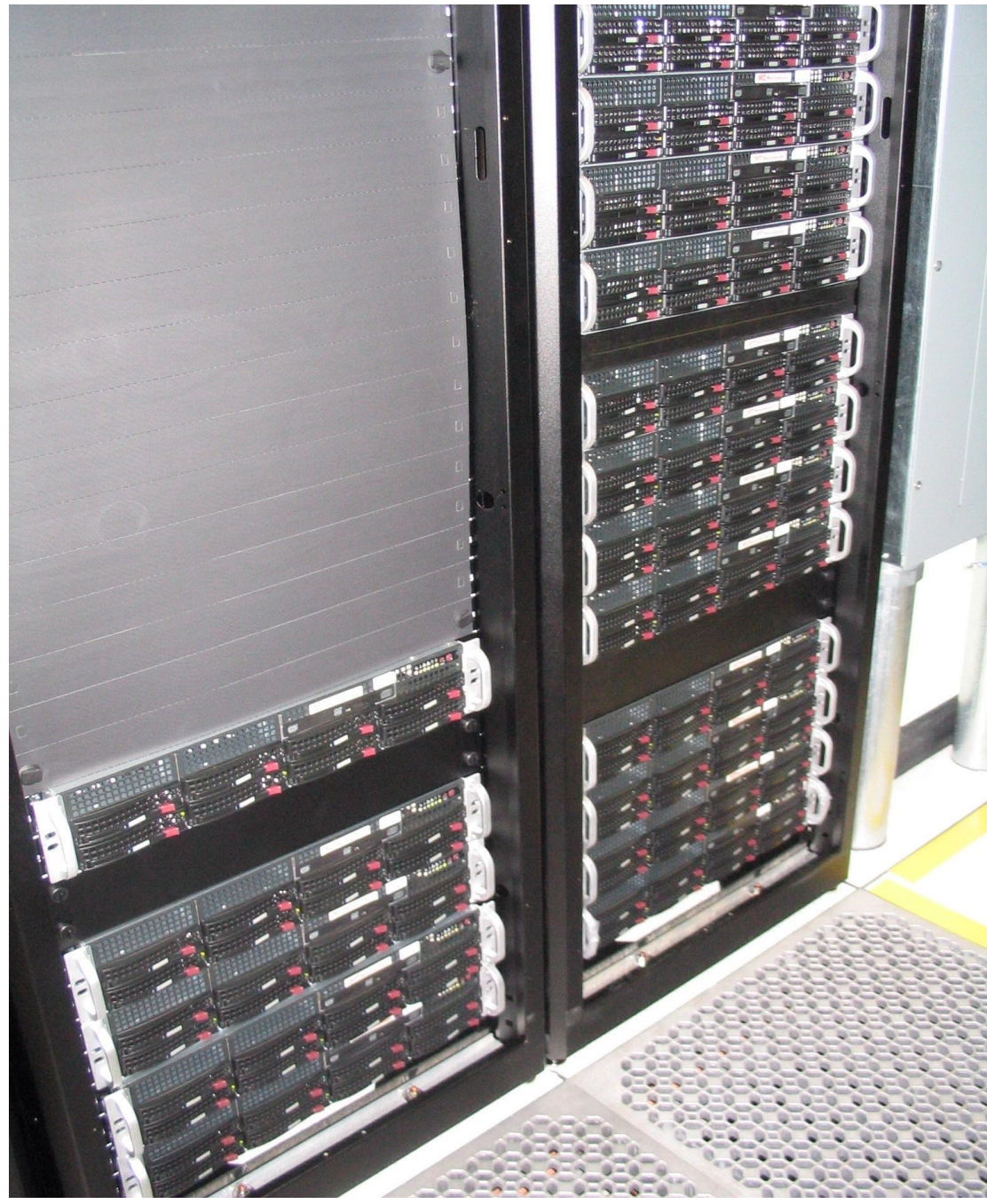
FermiCloud Production Hardware 23 nodes Dual Intel Xeon E5640 "Westmere" quad core CPU 24GB of RAM 2 x 300GB SAS system disks 6 x 2TB SATA data disk in RAID5 configuration High capacity LSI-1078 RAID controller, can source 300MByte/sec of data per machine. Dual GB Ethernet, 1 public network, one private. Mellanox "ConnectX2" Infiniband adapter.
